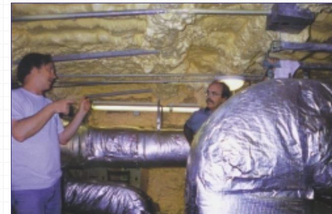
Wendell Porter of the University of Florida demonstrates, on a June day, how Icynene® keeps the unconditioned mechanical room at a comfortable temperature.
