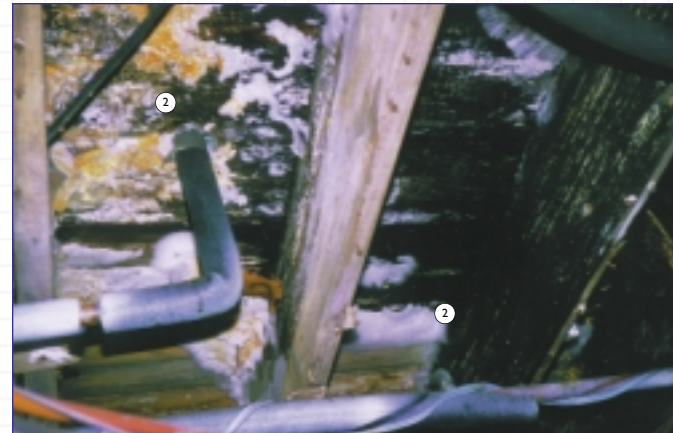
2) Various types of mold and mildew underneath the floors prior to remediation and installation of Icynene®
