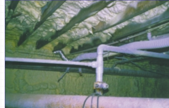
After 3.0 inches of Icynene® was applied underneath the floors and on the walls of the crawlspaces
